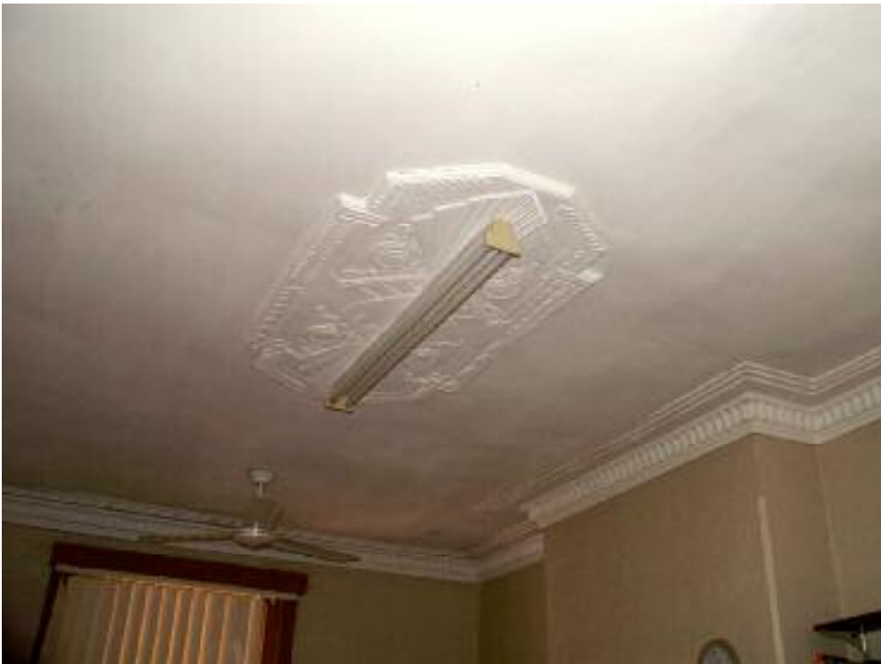
Photo 44 1 Surrey Street, Bassendean c.1893 residence: Interior view of c.1952 ceiling of the northwest front room. L Gray 7 June 2007
