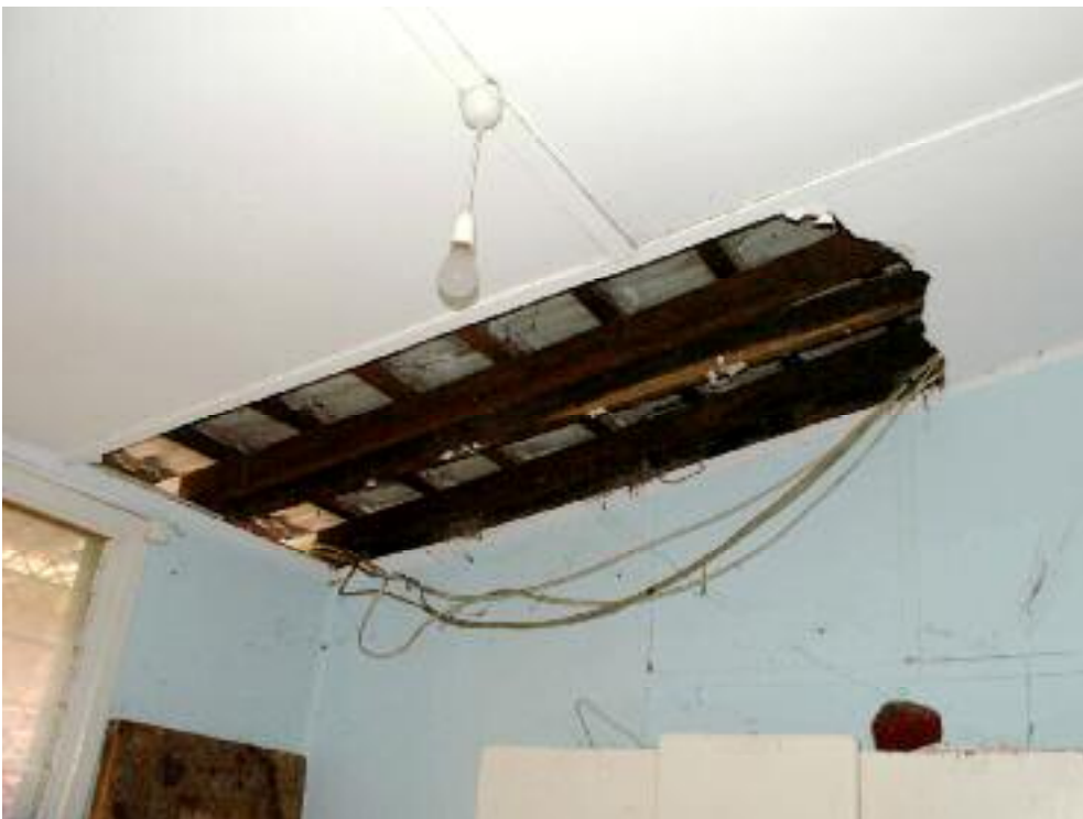
Photo 54 1 Surrey Street, Bassendean c.1893 northwest verandah room showing ceiling damage. L Gray 7 June 2007
