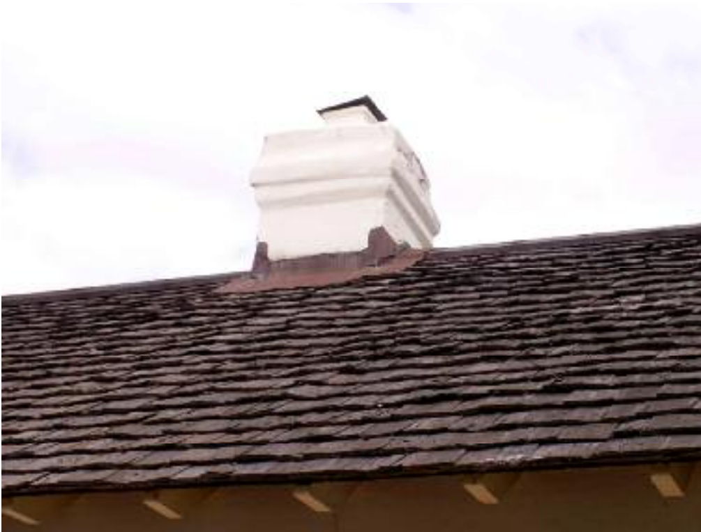
Photo 15 1 Surrey Street, Bassendean View of the shingle roof and rendered chimney. L Gray 7 June 2007
