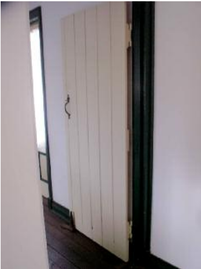
Photo 21 1 Surrey Street, Bassendean Interior connecting door to east room. L Gray 7 June 2007
