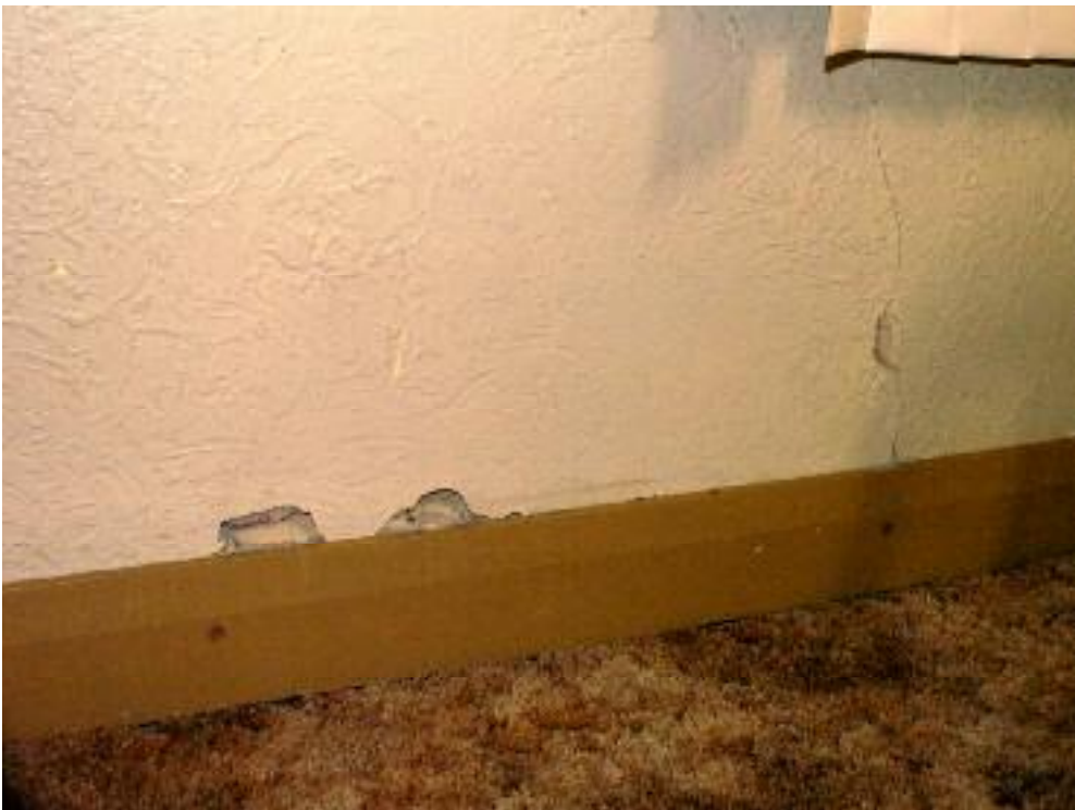
Photo 45 1 Surrey Street, Bassendean c.1893 residence: damage on the north wall of the northwest front room. L Gray 7 June 2007
