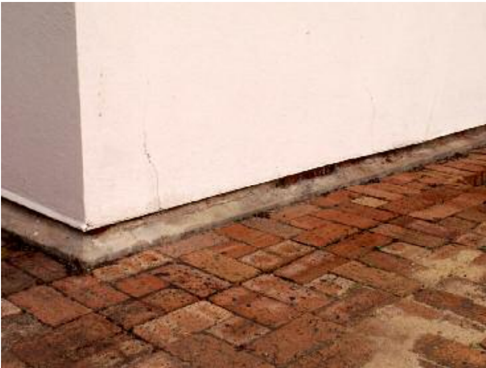
Photo 11 1 Surrey Street, Bassendean Edge perimeter detail of Pensioner Guard Cottage, showing cracking of the render. L Gray 7 June 2007
