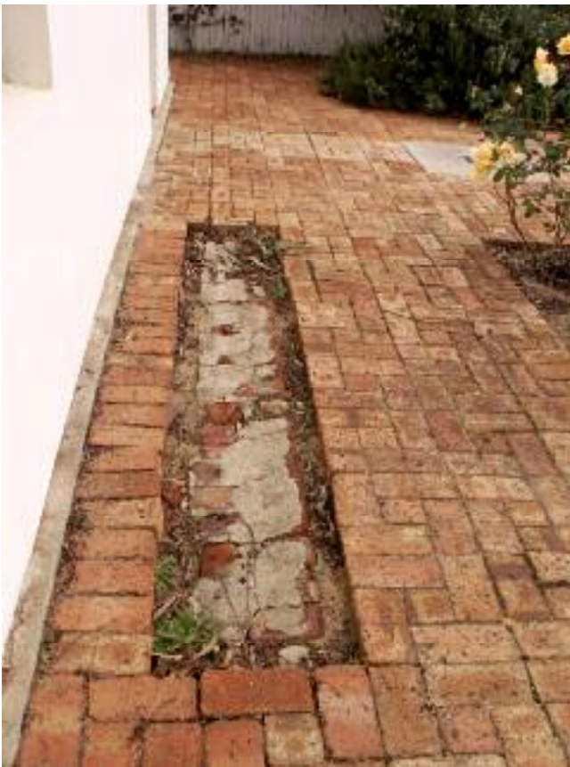
Photo 10 1 Surrey Street, Bassendean Drainage detail remnant at the front of Pensioner Guard Cottage. L Gray 7 June 2007
