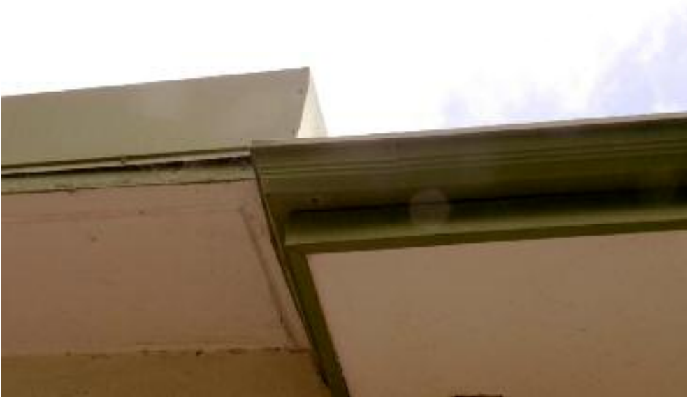
Photo 36 1 Surrey Street, Bassendean Roof connection on east side between c.1952 additions (left) and c.1893 roof. L Gray 7 June 2007
