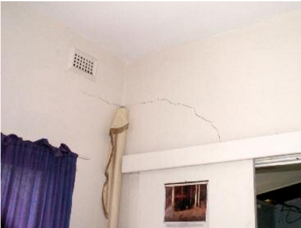
Photo 53 1 Surrey Street, Bassendean c.1952 addition: west room showing wall damage at connection to the c.1893 northwest verandah room. L Gray 7 June 2007
