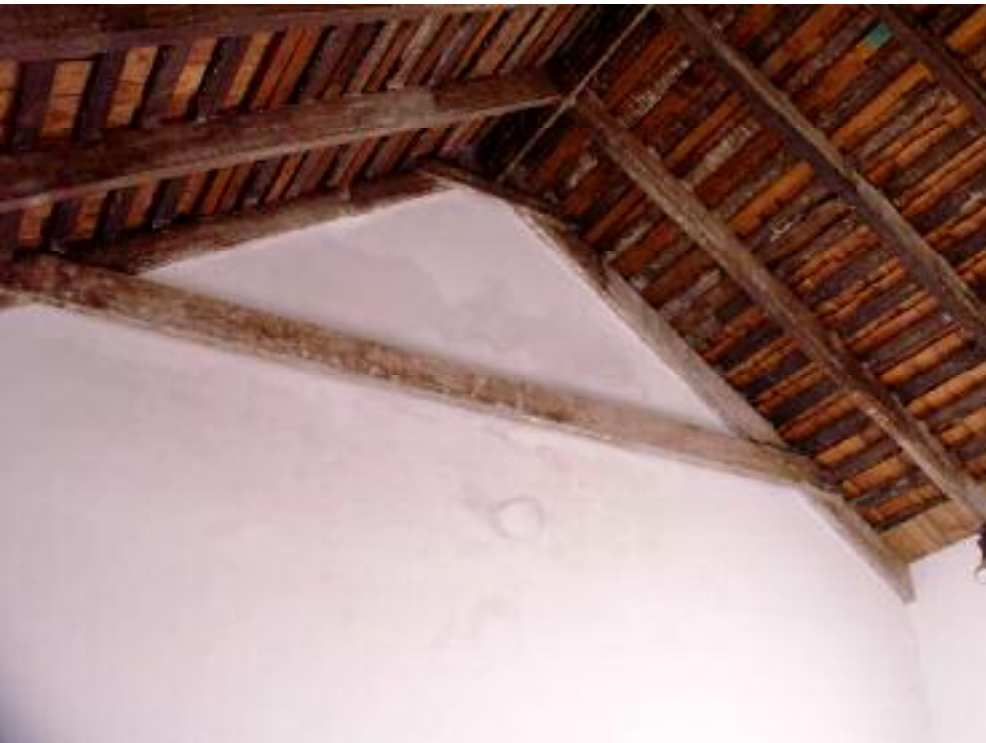
Photo 24 1 Surrey Street, Bassendean Interior view showing the original timber structure that formed the ceiling, with remnants of limewash evident on the timber. L Gray 7 June 2007
