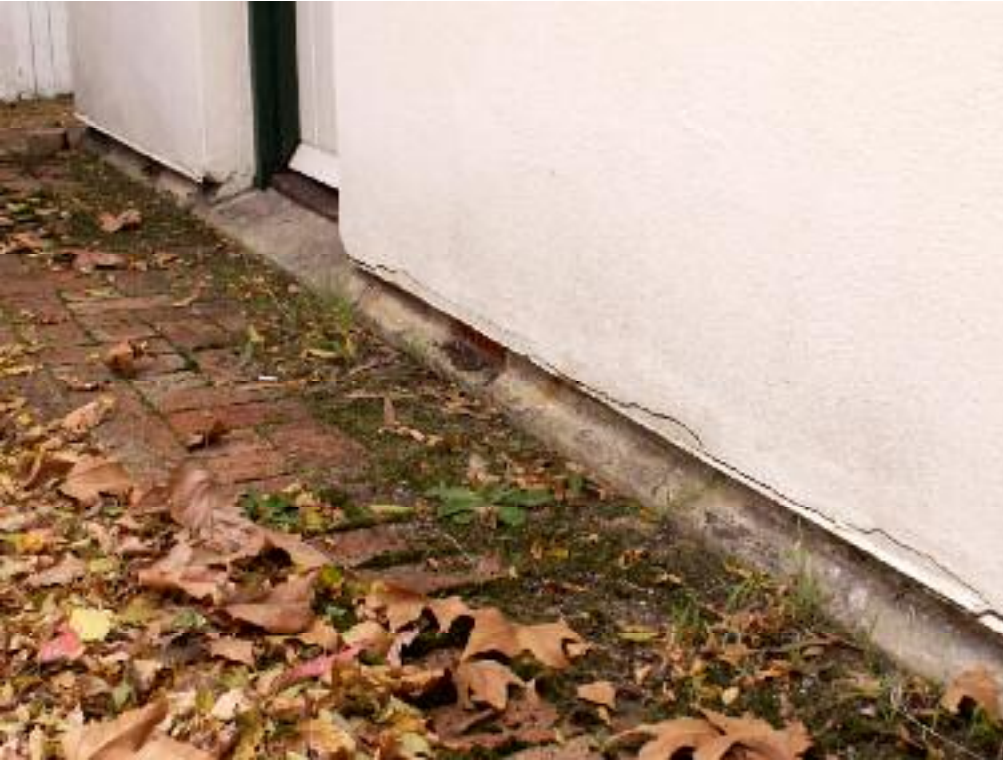
Photo 17 1 Surrey Street, Bassendean View of rear wall, showing cracking of render. L Gray 7 June 2007
