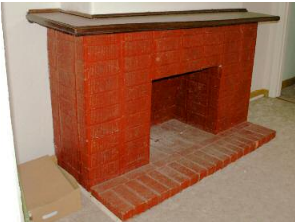
Photo 52 1 Surrey Street, Bassendean c.1952 addition: west room showing fireplace. L Gray 7 June 2007
