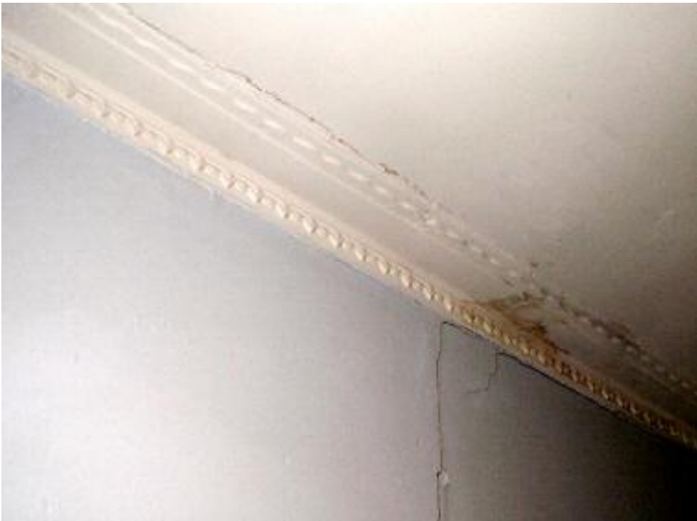
Photo 51 1 Surrey Street, Bassendean c.1952 addition: damaged ceiling and cracked wall. L Gray 7 June 2007
