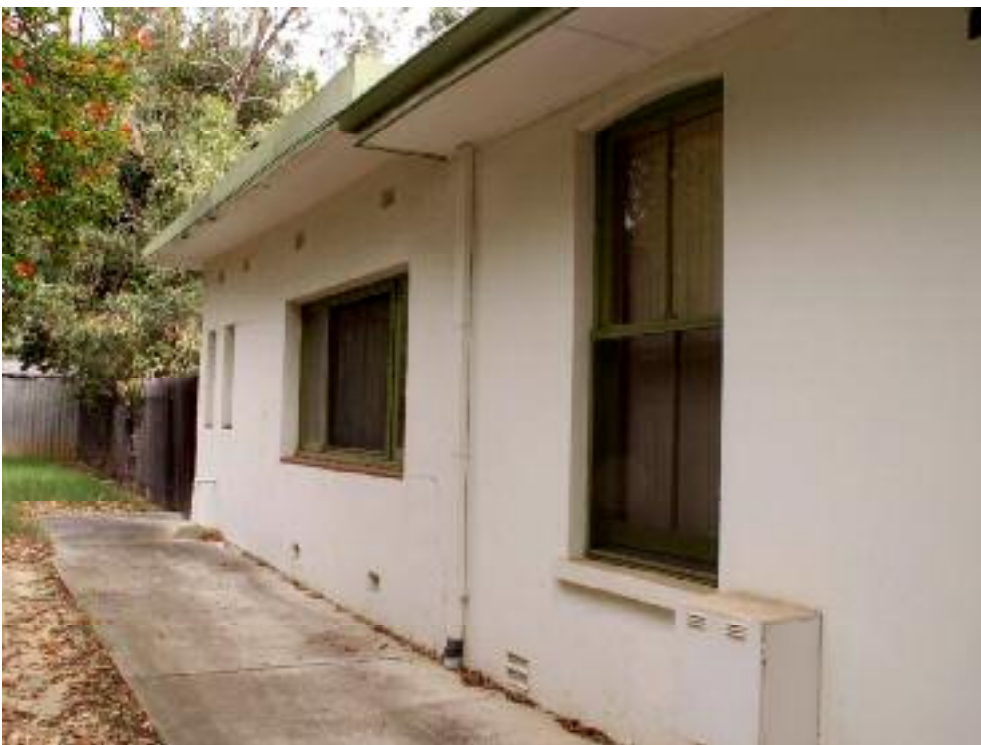
Photo 35 1 Surrey Street, Bassendean View looking south along the east side of c.1893 residence showing the c.1952 additions connection. L Gray 7 June 2007
